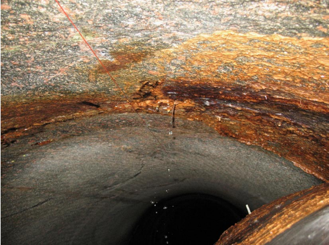
Water leakage at position 1.
