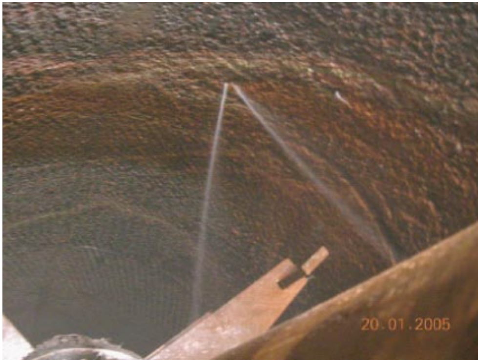
Figure 2-4. Picture from the initial situation with a sprinkling flow due to high pressure gradient / Bäckblom and Lindgren 2005/.
