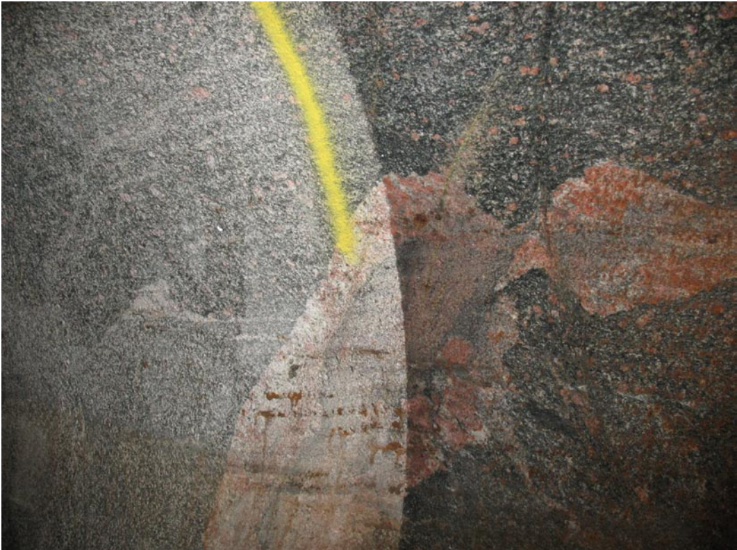
The rock wall after removing of the Mega-Packer showing the sealing effect.
