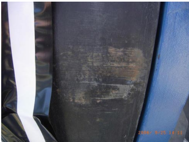
Figure 5-2. Minor scratches in one of the packers.
