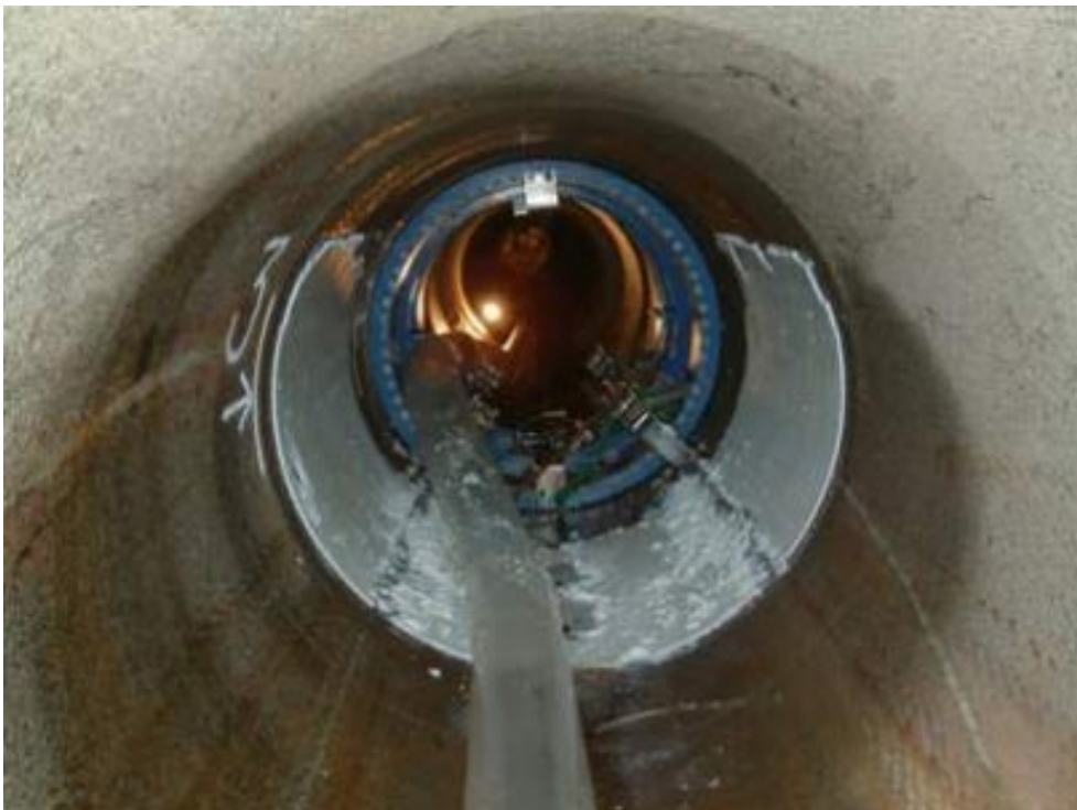
Figure 5-1. The unsuccessful filling of the gap in the Mega-Packer at position 3.
