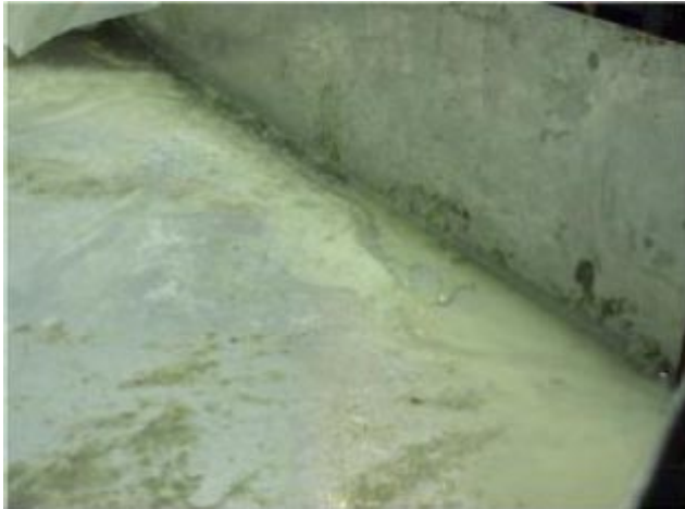
Figure A-14. Eroded bentonite pellet material in Test 8.
