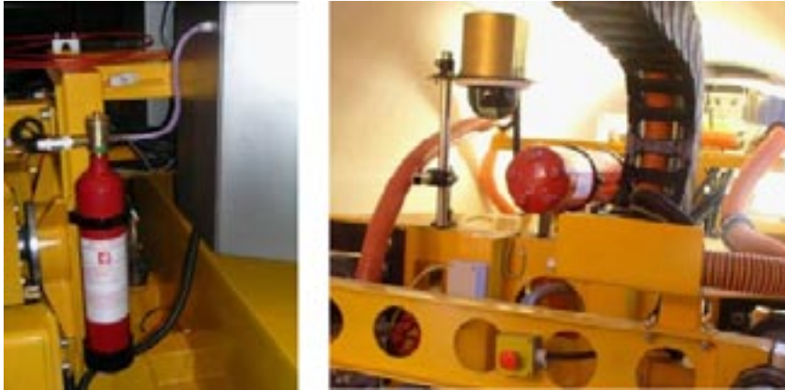
Figure 4-15. Fire extinguishers for electrical cabinet (left) and motors (right).
