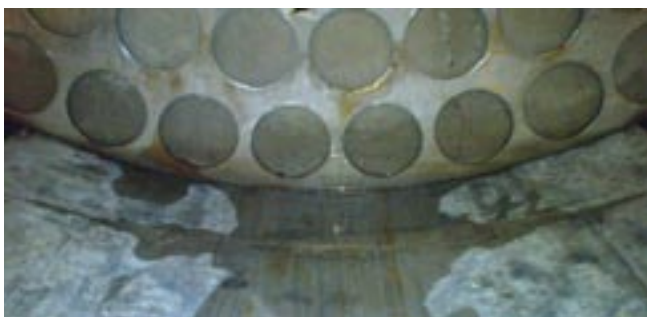
Figure 5-12. The picture shows that water has entered the slide plate and that the buffer has come in contact with water.
