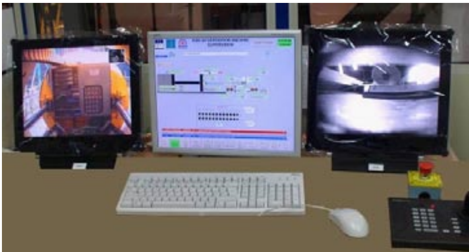
Figure 4-22. Equipment in the Control Room, (monitor for movable camera on the machine, right – monitor for HMI, middle – monitor for cameras on the slide plate, left).
