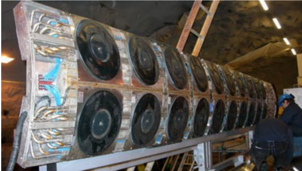
Figure 4-11. View of underside of the lift pallet during installation of water cushions.
