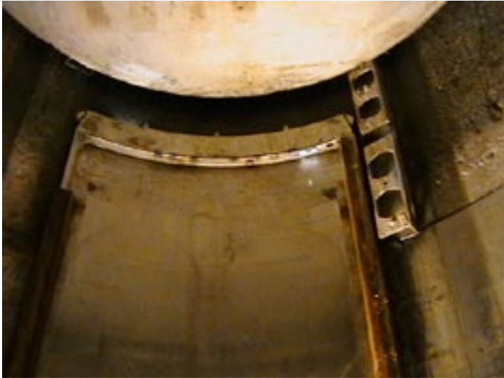
Figure 5-16. The feet have come loose from the Distance Block.
