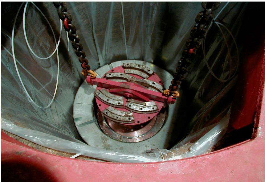
Figure 4-2 The canister is in place inside the column of bentonite cylinders in hole # 2. The gripping device has been made free from the lid and is being hoisted. The plastic, covering the walls, is installed for protection of the bentonite because of the long time between installation of blocks and backfilling of the tunnel. It will be removed before the slot is filled with bentonite pellets.
