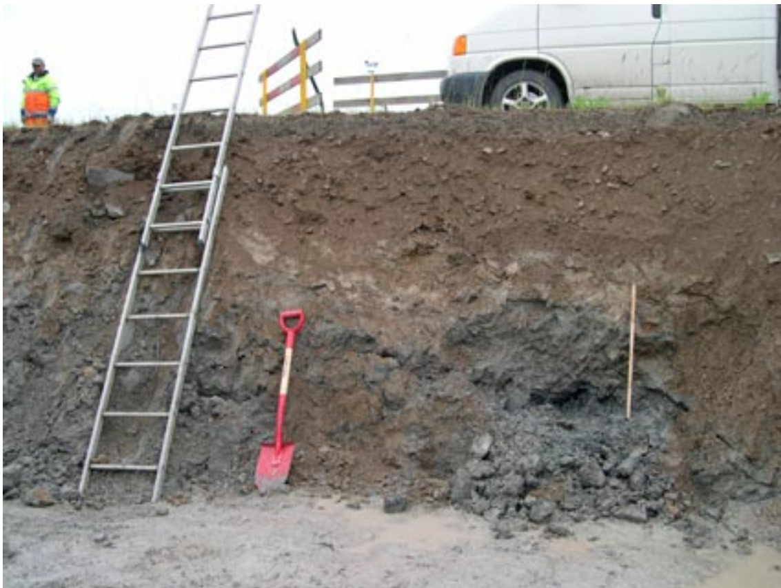
Figure 5-25. An excavation close to the reactor Forsmark 3 shows the artificial filling material consisting of blast bedrock material and re-deposited till (PFM004760).
