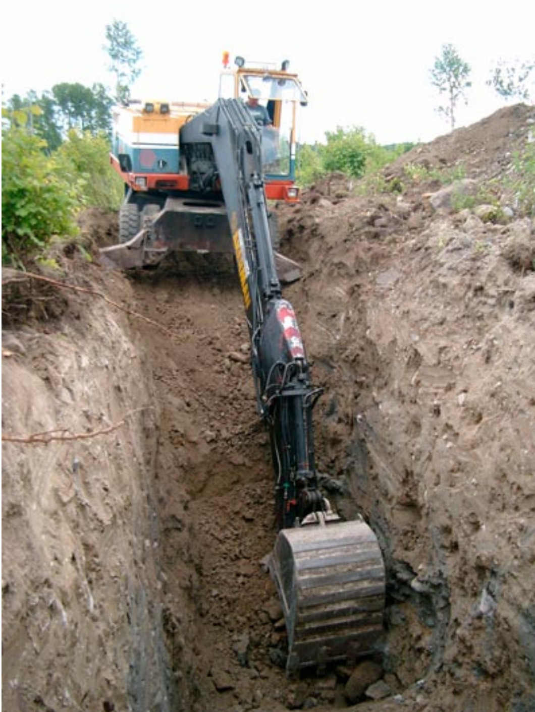
Figure 2-7. Stratigraphical investigations of the till were performed in machine-cut trenches. The walls were classified into lithological units. Samples were collected for grain size analysis and till fabric analysis was performed.
