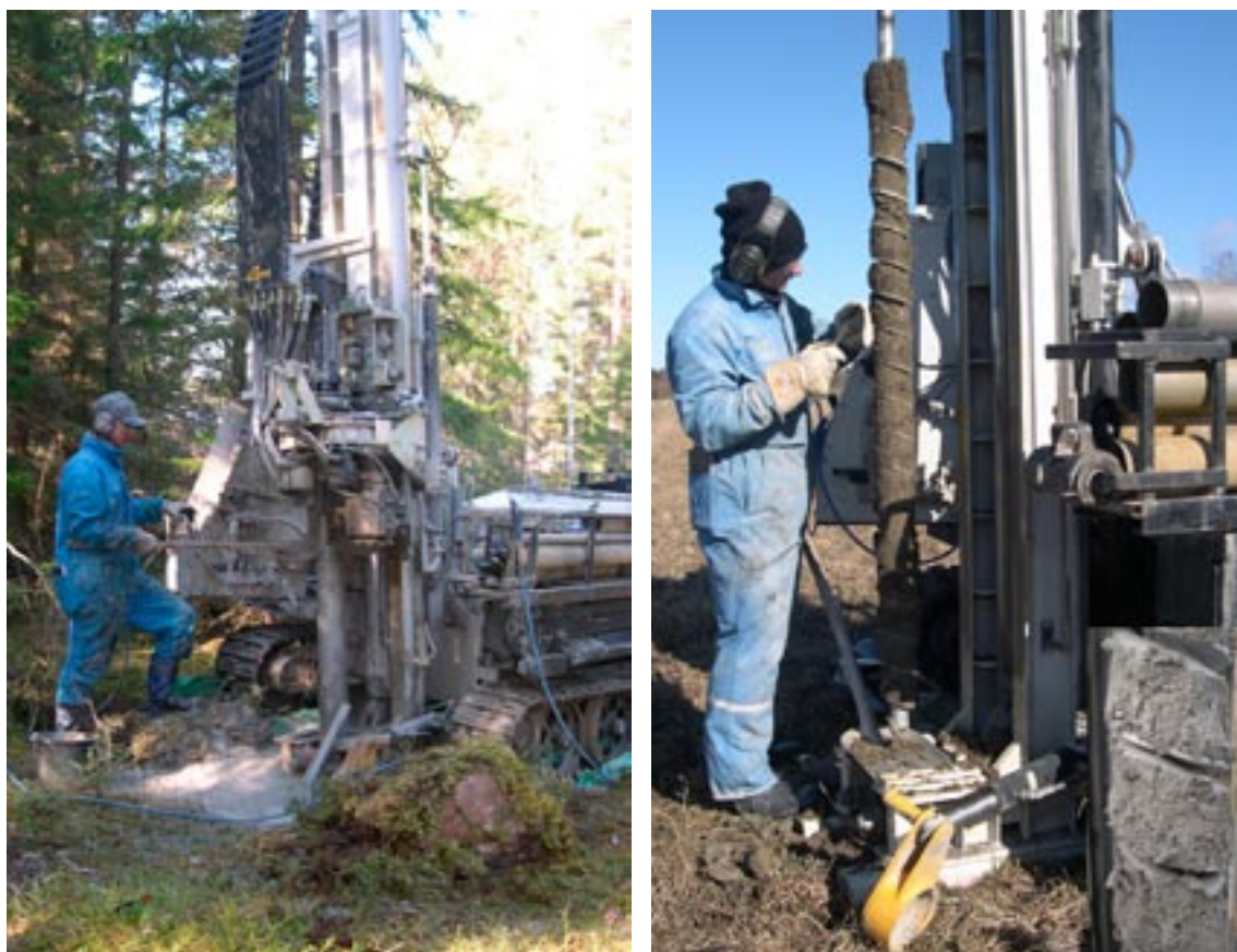
Figure 2-5. A) A majority of the HFM-corings were performed using percussion coring. The samples retrieved were often crushed and included bedrock fragments. B) Corings were performed using an auger drill during installation of groundwater monitoring wells (SFM-sites). The corings resulted in higher quality samples than those from the percussion corer. The photo shows clayey till obtained from a 4-m depth at Storskäret. Note the detail in the bottom right-hand corner showing the sediment after the cleaning of the sample.
