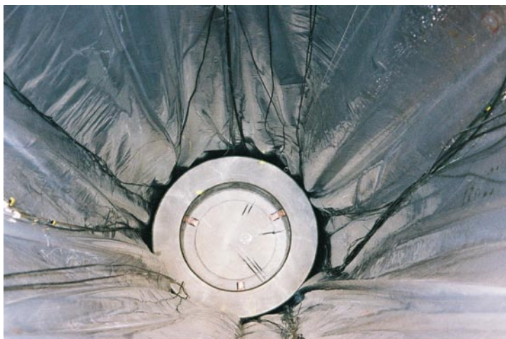
Figure 1-3. Photo taken after installation of the plastic sheet in the Prototype Repository project.
