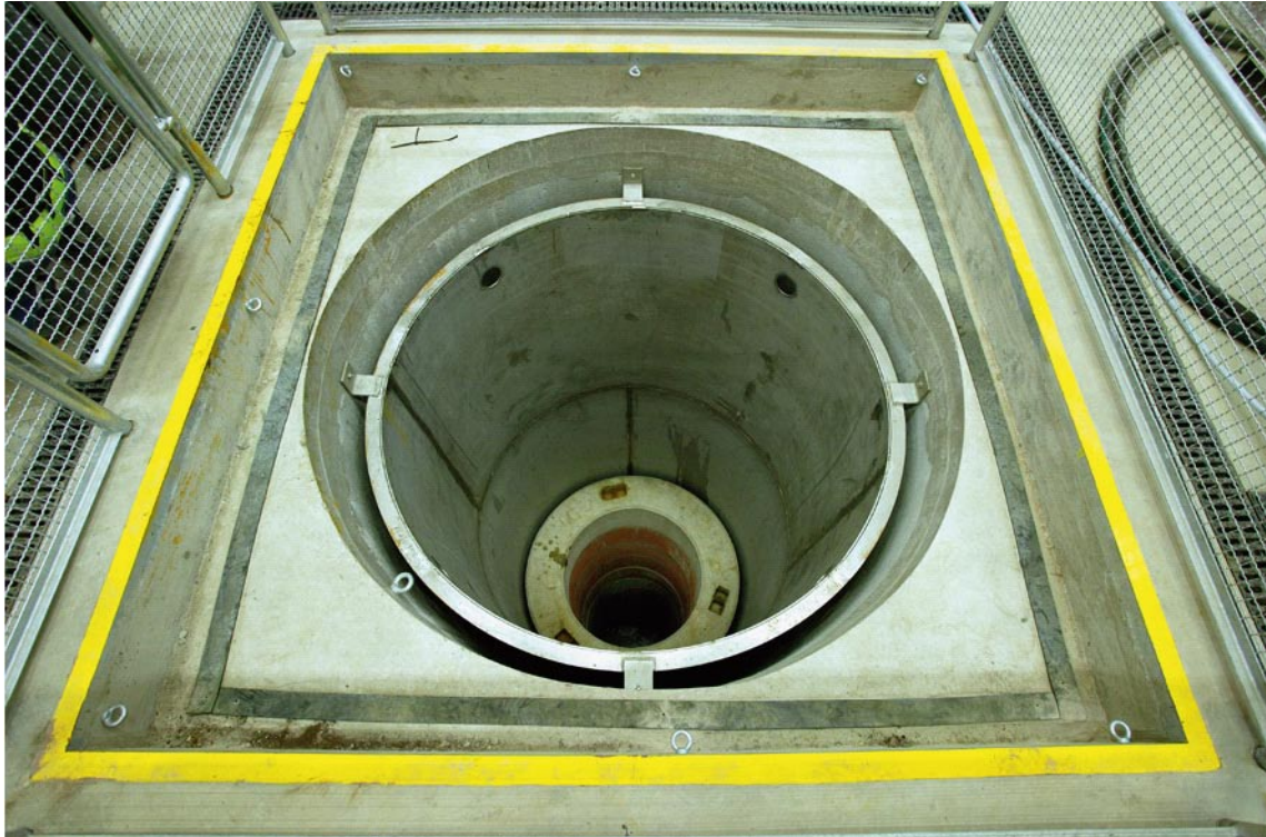
Figure 8-9. The "deposition hole" with buffer block column after completing the integrated experiment.
