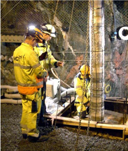
Installation of one of the three parcels illustrating the mixing of the different compacted buffer discs.
