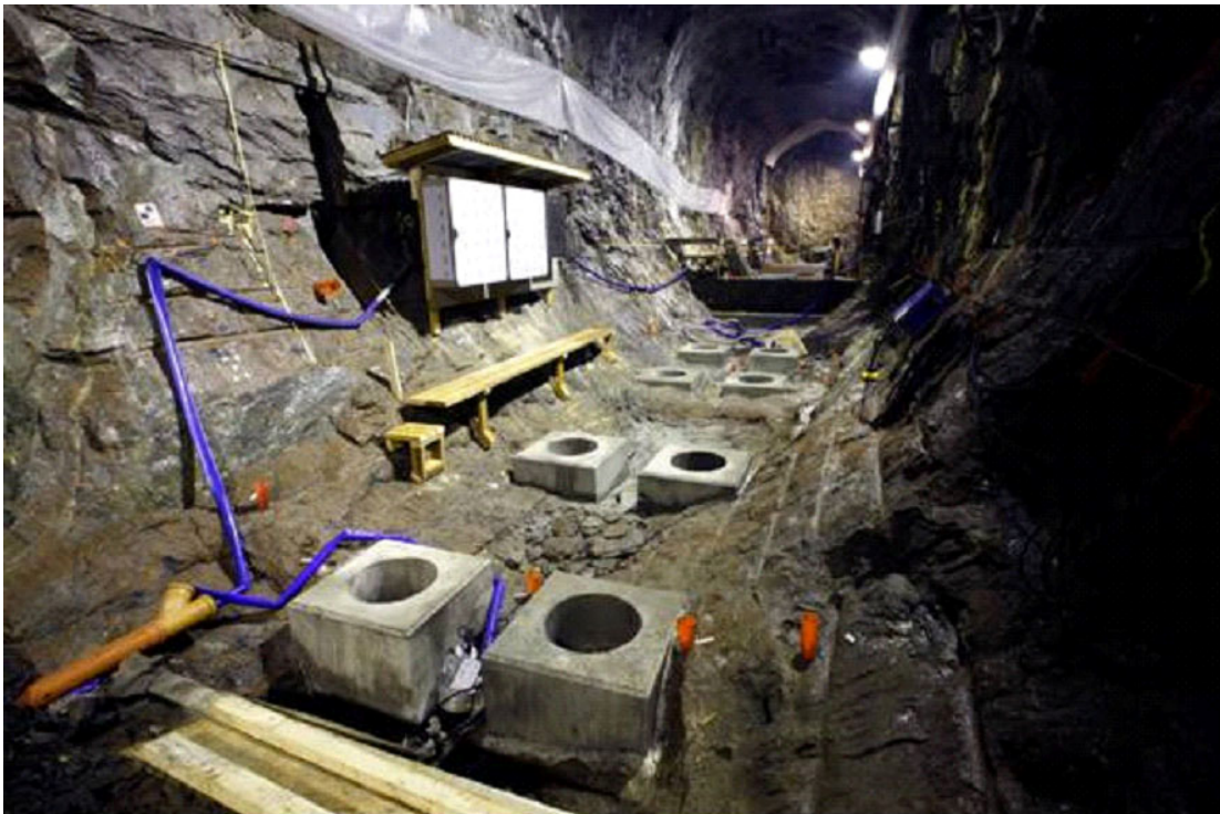
Figure 2-1. Installation of test equipment in Tasq-tunnel for the project Counterforce Applied to Prevent Spalling.
