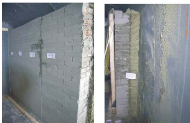
Figure A-17. Evidence of early seepage through block assembly in Test 8.
