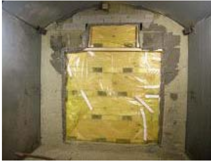
(a) Wet downstream face
