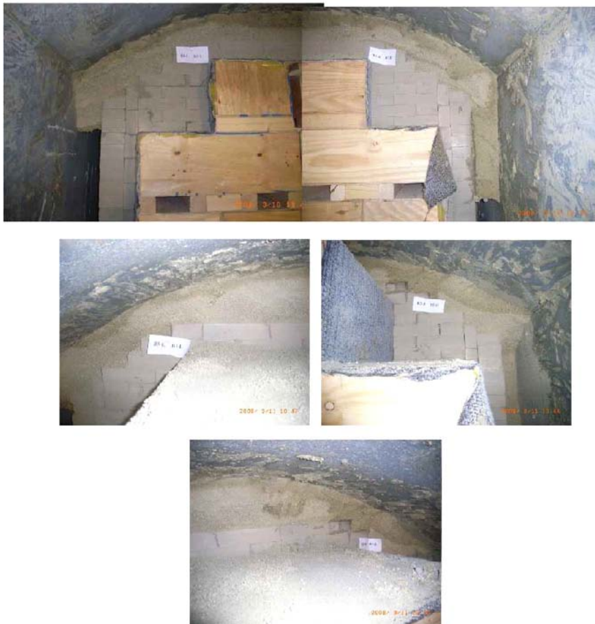
Figure A-11. Wetting along crown of Assembly 3 (Tests 5, 6).
