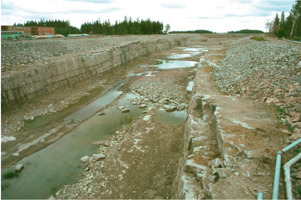
Figure 5-14. Picture from the construction of the 13 m deep and more than one kilometre long canal between the Baltic Sea and the nuclear power reactors in Forsmark. Horizontal fractures/sheet joints are encountered along the entire excavation. The sheet joints follow the undulations of the bedrock surface implying that many of them do not outcrop, but stay below the bedrock surface as this dips under the Baltic Sea. There are several “horizons” of extensive sheet joints on top of each other according to the hydraulic interference tests. The picture is taken from the southern side of the canal where the bridge crosses the canal between drill sites 7 and 8. Photograph by G Hansson.
