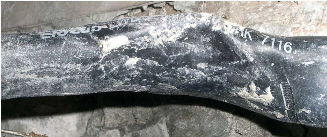
Figure 11. The power cables show damages from the bentonite swelling pressure at several positions.
