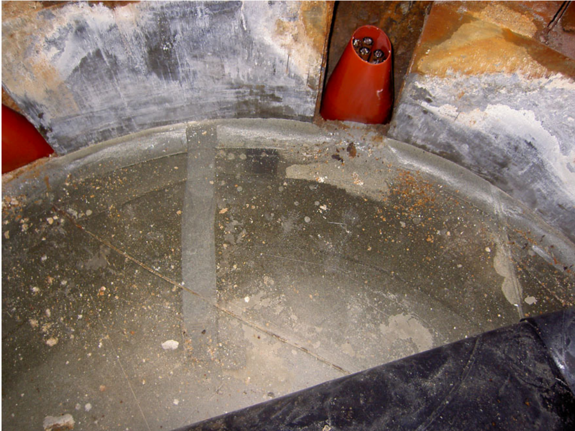
Figure 7. The upper buffer surface as it looked when the rubber mat was first lifted. No damage on the buffer could be found.
