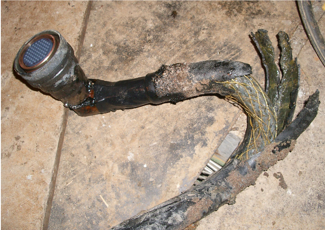
Figure 12. Damage on the heater power cable shield. The damage is located between the canister lids and close to the gisma connector.
