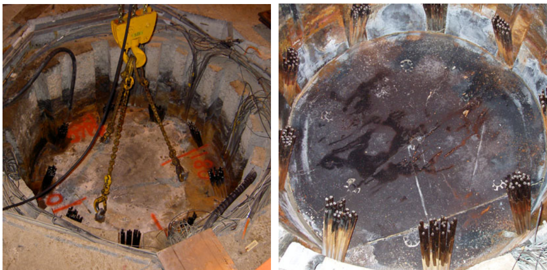
Figure 6. Lifting the concrete block. The lifting was straightforward and no issues encountered. To the right the rubber mat under the concrete plug is shown.
