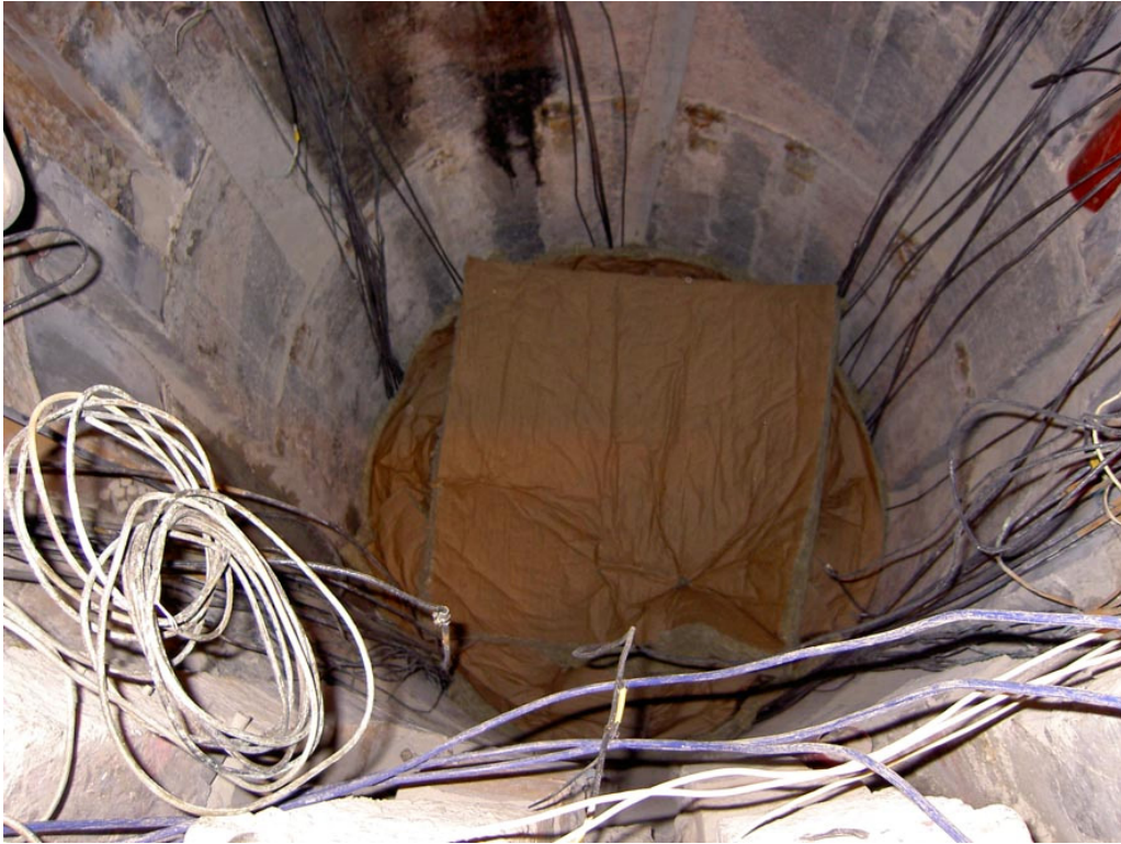
Figure 14. New cables were fitted and the heaters restarted. No issues were encountered during this test. The deposit hole was insulated to prevent too much ventilation and temperature loss.
