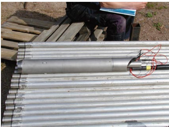
Photo 5. Positioner, bottom end of down-in-hole string.
