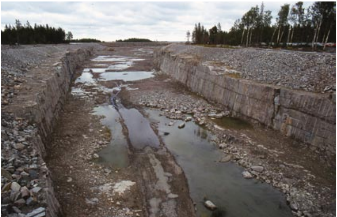
Figure 2-7. Observed near horizontal and subvertical fracturing along the Forsmark cooling water inlet channel.
