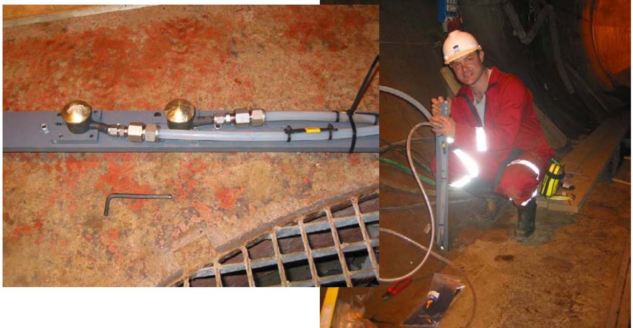
Figure 4-13: Top: Schematic diagram of the locations of all transducers on a single frame. Left: Photo of a section of the transducer assembly. Right: The transducer assembly during installation.
