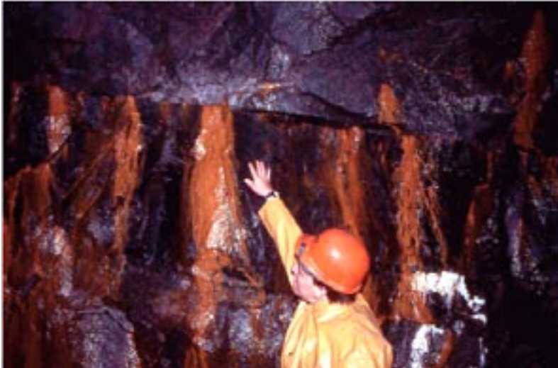
Figure 3-1. Channelling seen in the Bolmen tunnel as precipitates of iron oxides.
