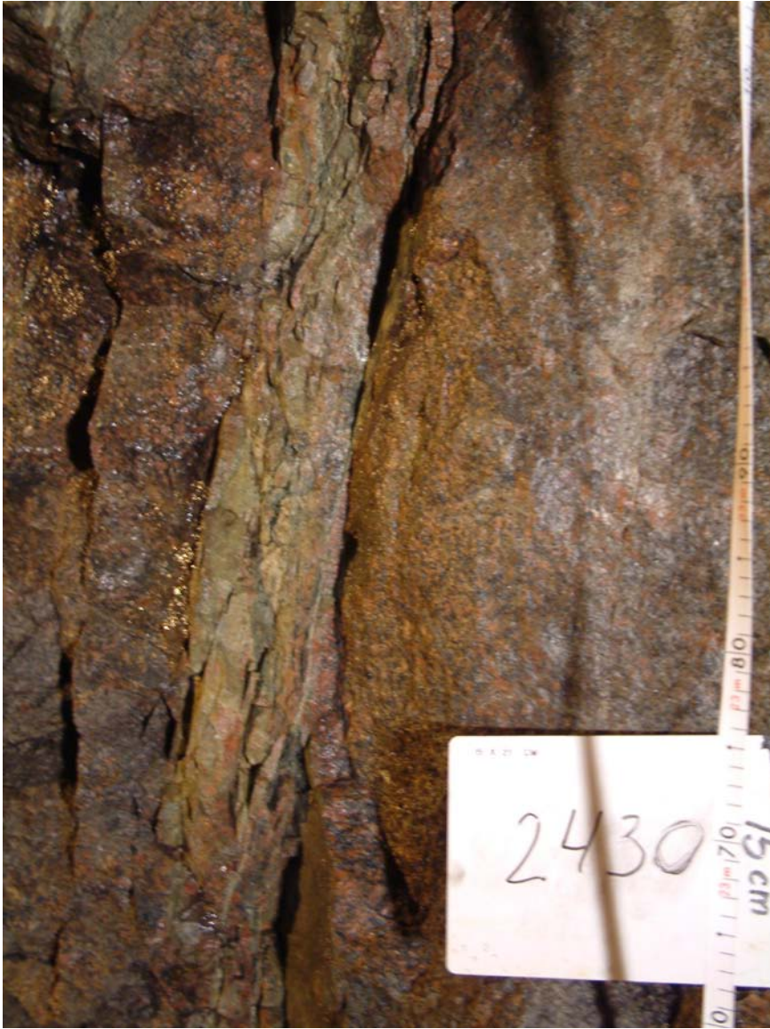
Figure A1-4. Fault visible in tunnel section 2/430 m.
