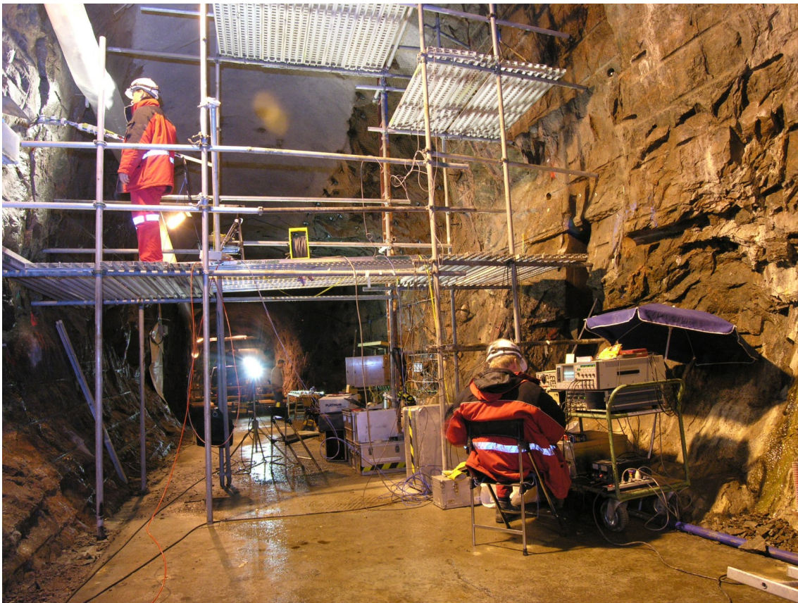
Fig. 1. Ultrasonic measurements with the BGR mini sonic probe in the TASQ tunnel. View towards the entrance of the tunnel.
