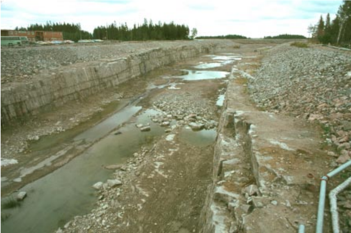
Figure 2-22. Picture from the construction of the 13 m deep and more than one kilometre long canal between the Baltic Sea and the nuclear reactors. The horizontal fractures/sheet joints are encountered along the entire excavation. There are several “beds” of more or less extensive sheet joints on top of each other. The picture is taken from the southern side of the canal where the bridge crosses the canal between drill sites 7 and 8, see Figure 2-1.
