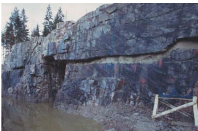
Figure 2-15. Photograph of a sediment filled horizontal sheet joint encountered during the excavations for the nuclear power reactors in Forsmark /Carlsson 1979/.
