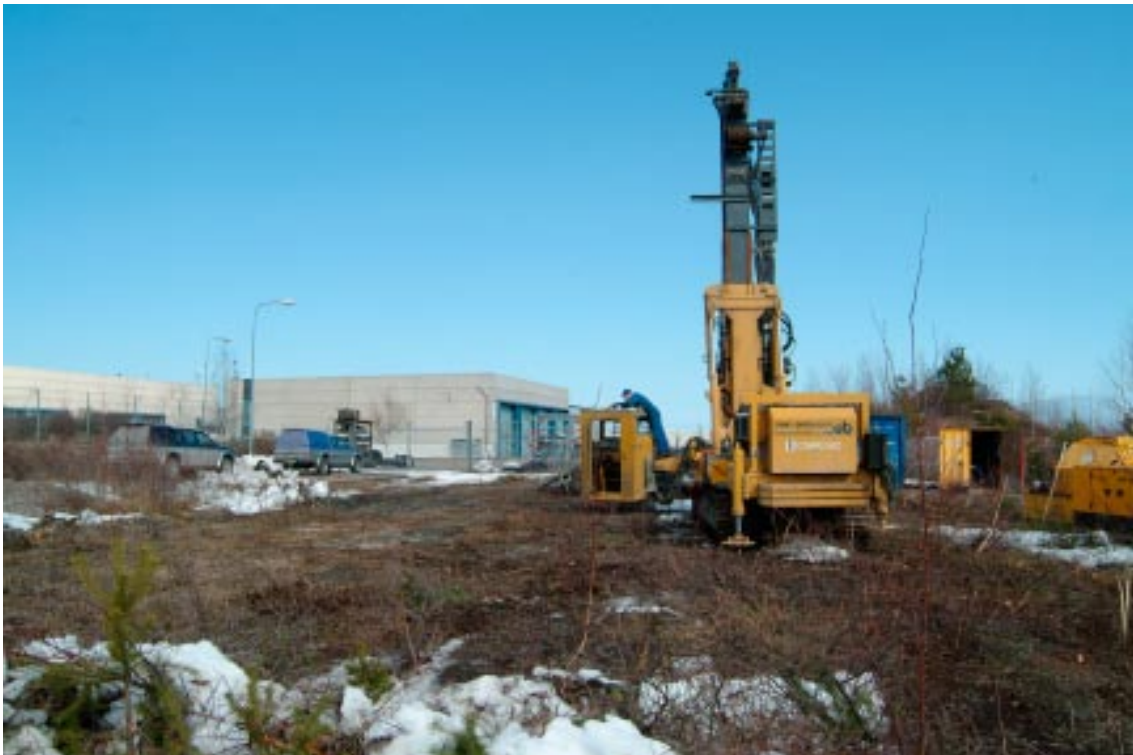
Figure 3-1. The Comacchio 1500 S drilling machine at HFM33, close to drill site DS11.
