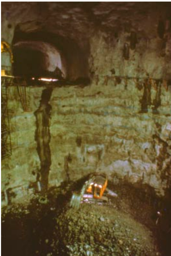
Figure 6-7. The excavation sequence of the silo, SFR, a. (1) Excavation of the dome. (2) Long-hole drilling and blasting. (3) Bench blasting. /Schutz 1986/.
