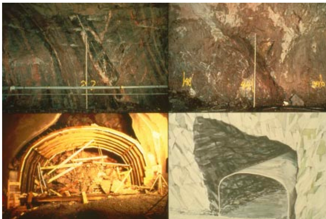
Figure 9-1. Illustration of the difference in rock mass conditions within the Singö deformation zone between Forsmark 1 and 2 tunnel (upper pictures) and the Forsmark 3 tunnel (lower pictures).
