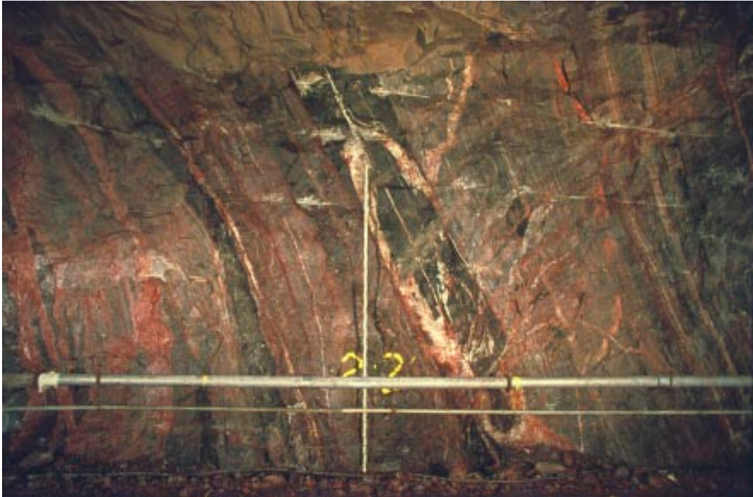
Figure 4-4. Brecciated metagranite within the Singö deformation zone with numerous veins of quartz and calcite, Forsmark 1 and 2 tunnel /Carlsson and Olsson 1977/. Photo G Hansson/N.
