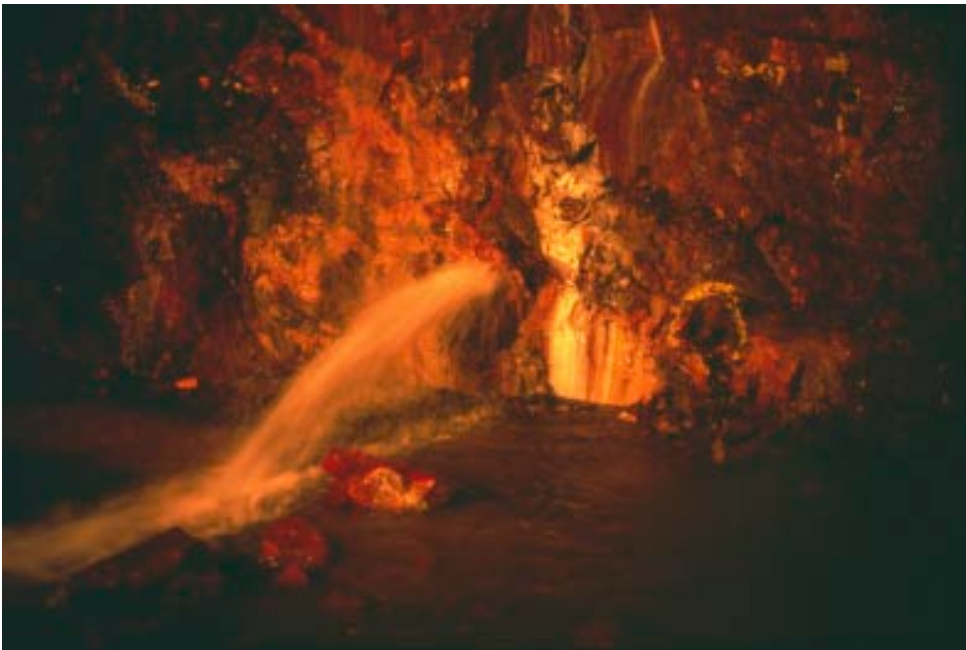
Figure 4-8. The water leakage in steep dipping fractures as distinct inflows at a lower boundary of the fracture, Forsmark 3 tunnel.
