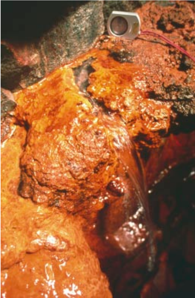
Figure 4-7. Water inflow from an aperture in a horizontal fracture. Large quantities of iron and manganese sediments, Forsmark 1 and 2 tunnel. Photo G Hansson/N.
