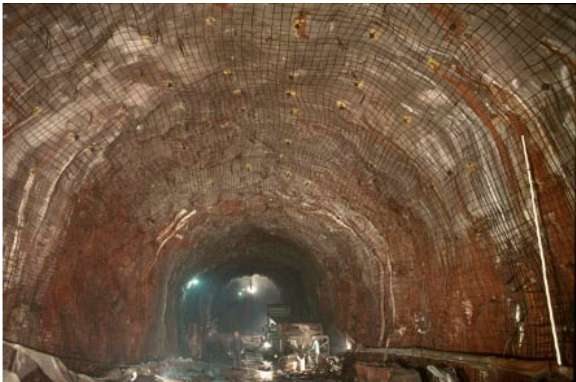
Figure 7-10. Rock support in rock class 4. The wire mesh was later covered by shotcrete. Forsmark 1 and 2 tunnel.
