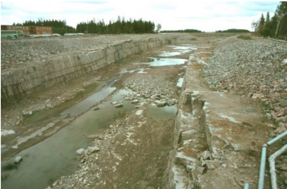
Figure 7-2. a. Observed horizontal and sub-horizontal fracturing along the inlet canal for cooling water to Forsmark nuclear the power plants. b. Continuous horizontal fractures in the northern wall of the inlet channel. Photo G Hansson/N.
