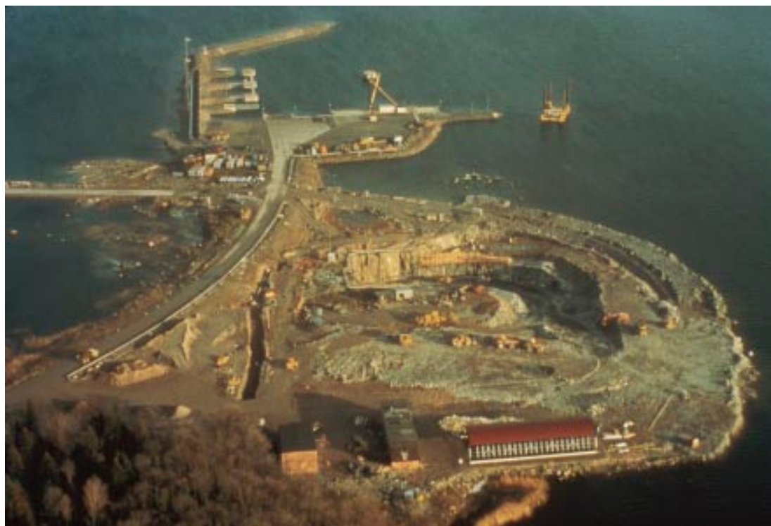
Figure 5-3. The location of the portaling of the SFR access tunnels on the rocky islet, Österblänkarna. Photo G Hansson/N.
