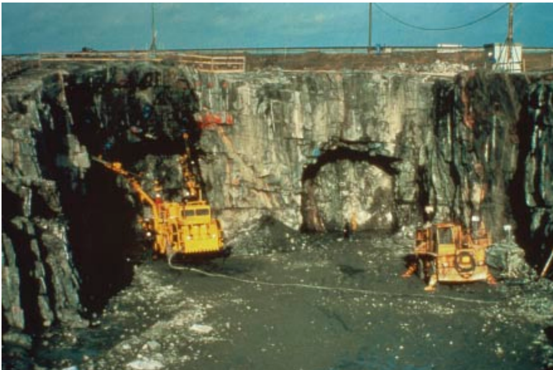
Figure 5-4. The access tunnels of the SFR are sited parallel to each other with a short distance in between (15 m).
