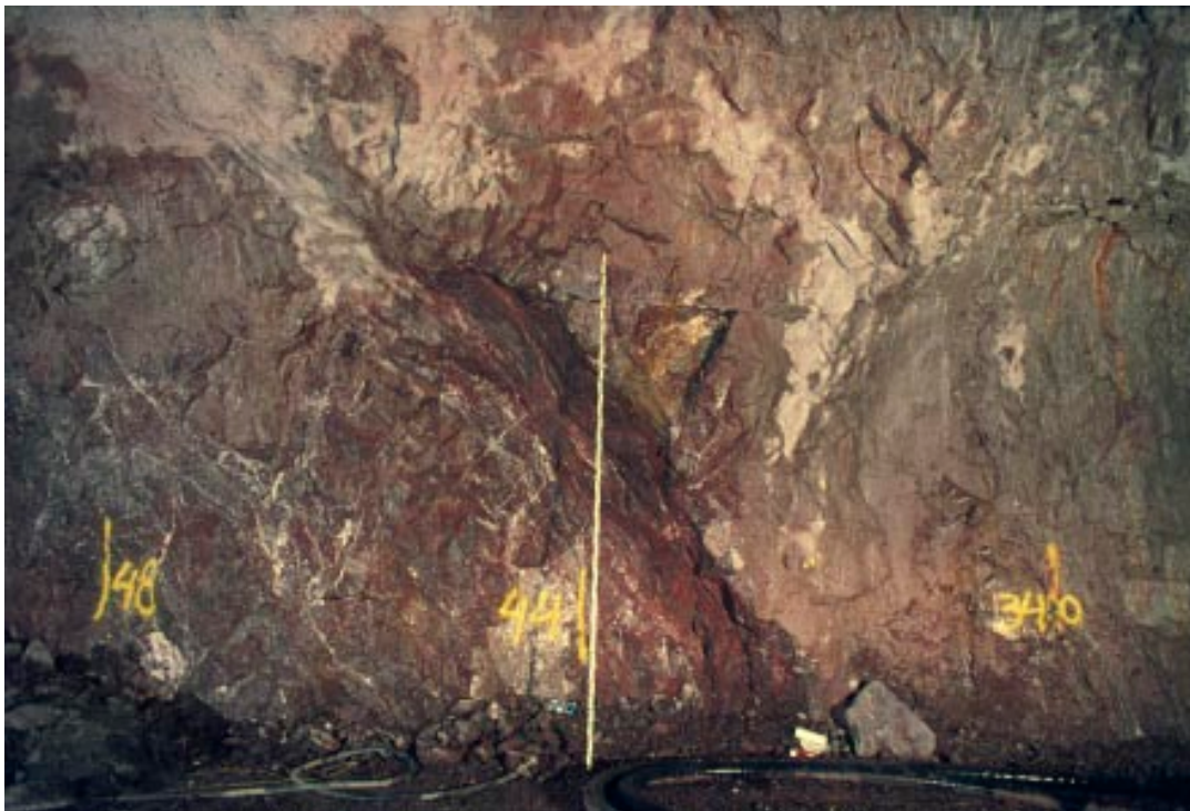
Figure 4-3. Clay-filled joint in brecciated metagranite within the Singö deformation zone, Forsmark 1 and 2 tunnel, /Carlsson A, Olsson T 1977/. Photo G Hansson/N.
