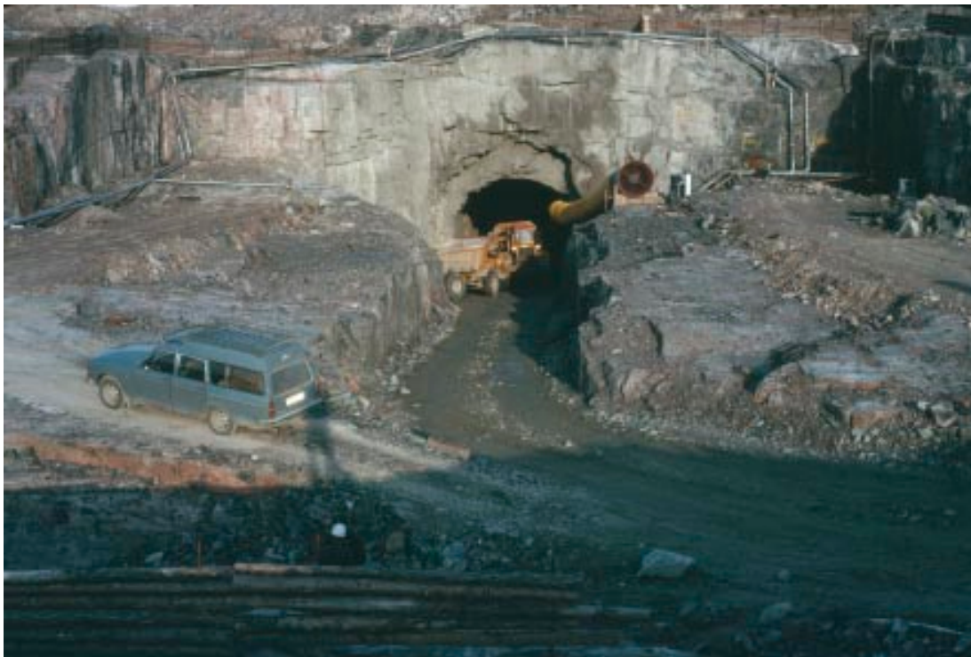
Figure 3-12. A view of the portaling of the recirculation tunnel of Forsmark Unit 3, where rock spalling occurred after some metres of excavation. Photo G Hansson/N.
