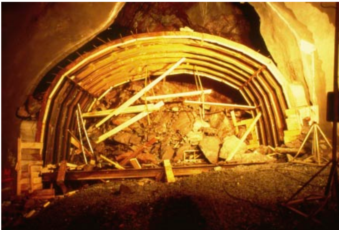
Figure 4-11. a. The steel arch placed in position within the overbreak area in section 2/545 in the Singö fault, Forsmark 3 tunnel. b. Further rock fall occurred after the erection of the steel arch; section 2/545 in the Singö deformation zone, Forsmark 3 tunnel.
