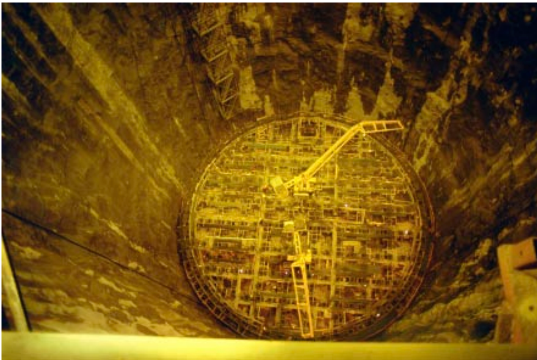
Figure 5-5. Slip-forming work, SFR. The photo shows the slip-forming work viewed from the top of the silo. Photo G Hansson/N.
