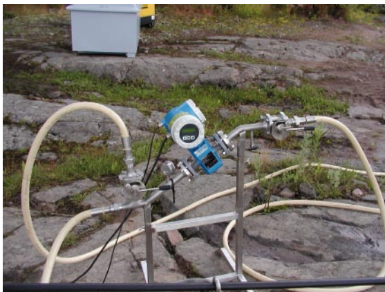
Photo 3. Surface flow meter for measuring total flow rate.
