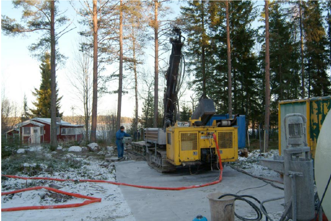
Figure 3-2. The Nemek 710 TE percussion drilling machine employed for drilling percussion boreholes HFM24 and SFM0080 at drill site DS10 as well as HFM28 at drill site DS9.
