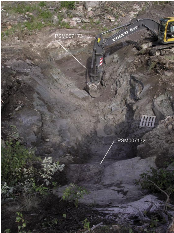
Figure 5-4. Profile 3. Looking to north-west. Observation points are marked with id-number in picture.
