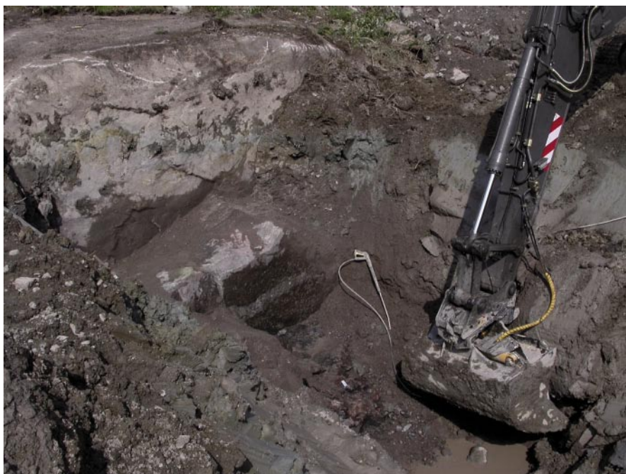
Figure 5-5. North-western part of the trench at Profile 3. A fractured, complex rock mixture of strongly altered and red stained, quartz monzodioritic Ävrö granite, fine grained red granite and fine grained mafic rock.
