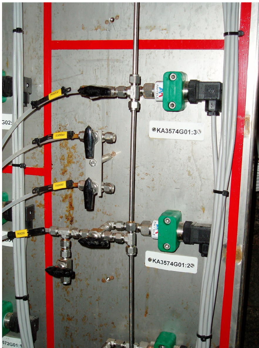
Figure 4-2. Pressure transducers connections
