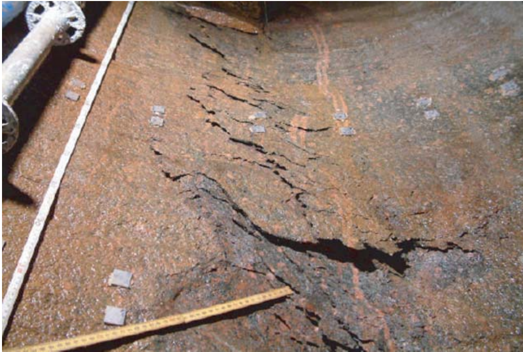
(a) Spalling slabs
