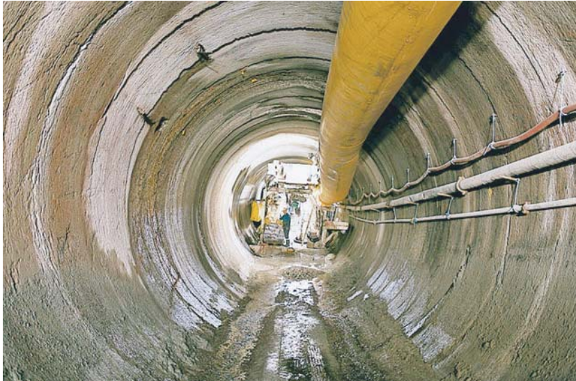
Figure 5–8: Example of the 5-m-diameter TBM tunnel profile at Äspö at a depth of 450 m. No spalling was observed in the TBM tunnel
