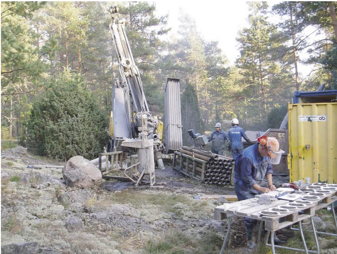
Figure 3-1. Drill site HLX36, the drill rig and equipment for preliminary geological mapping.
