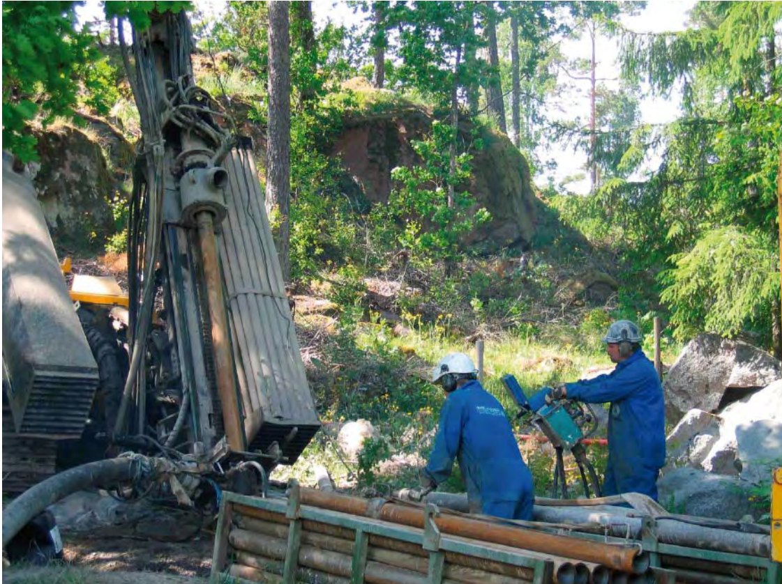
Figure 4-2. Drilling rig and crew drilling percussion borehole HLX34 in the north-western part of the Laxemar subarea.
