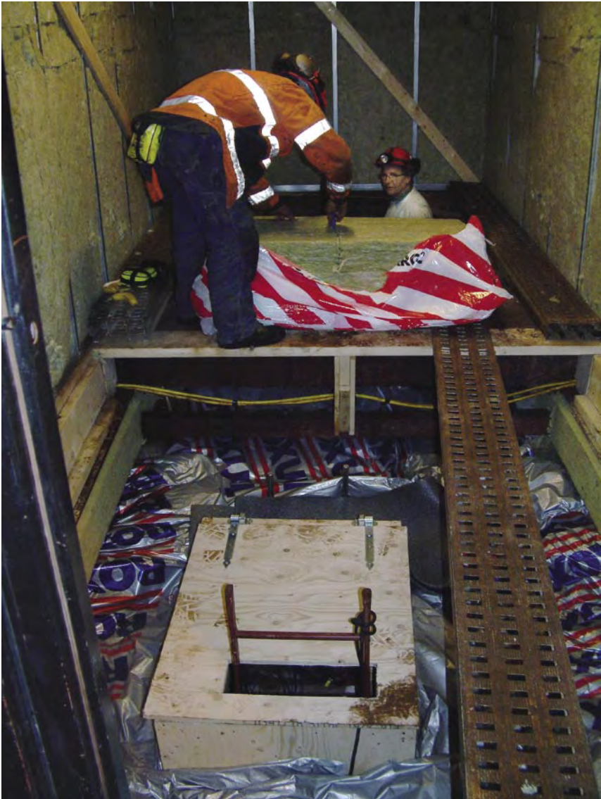
Figure 3-5. Photograph of rock floor insulation and the insulated plywood construction placed on top of the open hole (DQ0063G01) to prevent air convection.
