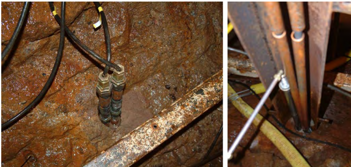
Figure 3-3. Photograph of the packer pipe and the heaters coming up from KQ0065G03 (Figure 3-4). The left photograph is the typical installation of heaters in the other three holes.
