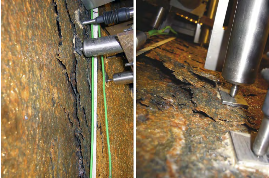
Figure 5-43. June 2. Photograph of spalling/fracturing at positions #3 (left) and #10 (right).
