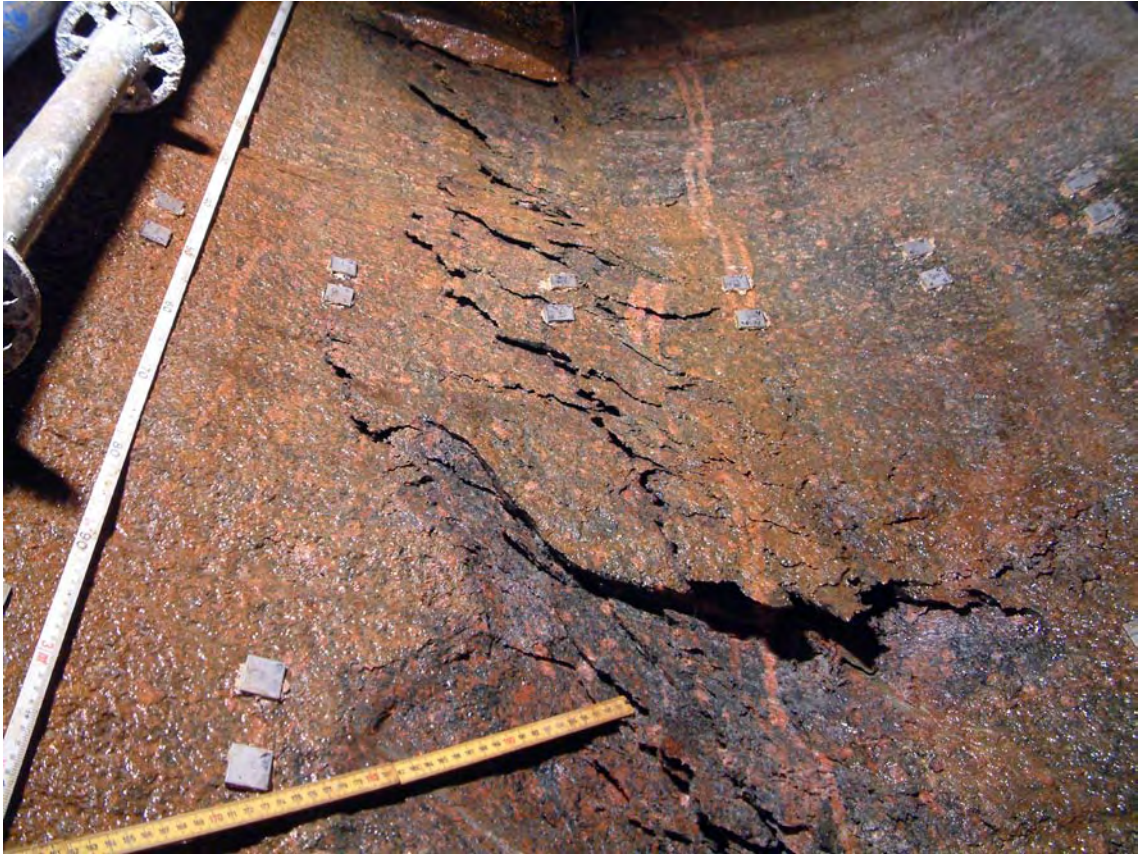
Figure 5-63. Photograph of the slabs with a free left surface and the right side attached to the rock wall. The depth at the bottom of the photograph is 3 m.
