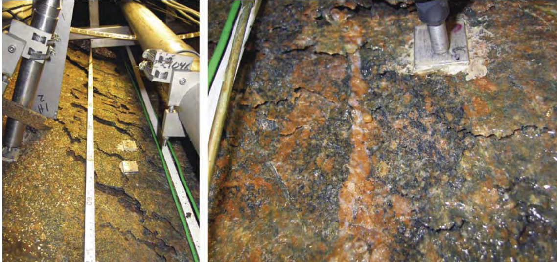
Figure 5-50. June 23. Photographs of spalling/fracturing at position #3 on the 2.5 m level (left) and at position #10 on the 3 m level (right).
