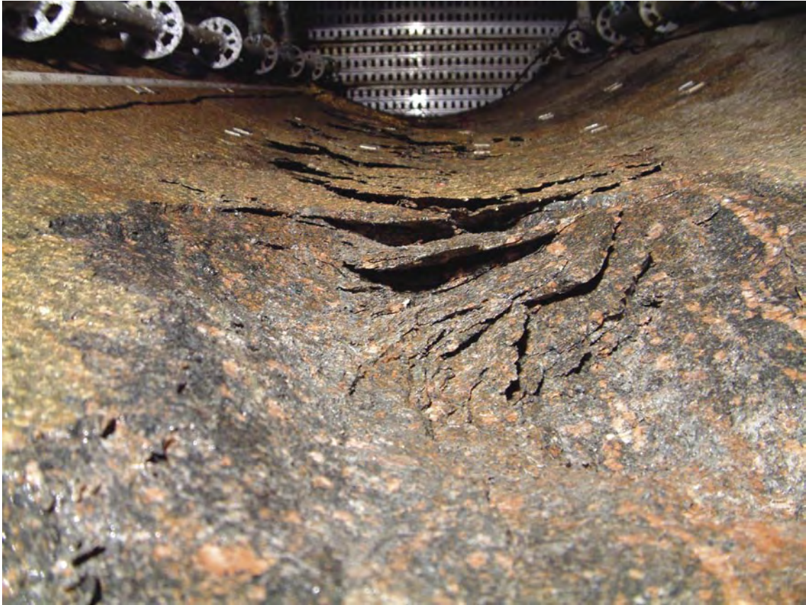
Figure 5-61. Photograph taken from below of chips at 3.7 m and up. The dilatation and curvature of the slabs can be seen.
