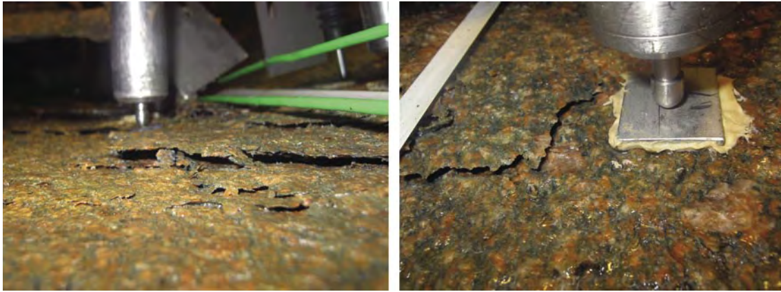
Figure 5-39. May 25. Photograph of the short-range sensors at positions #3 (left) and #4 (right).
