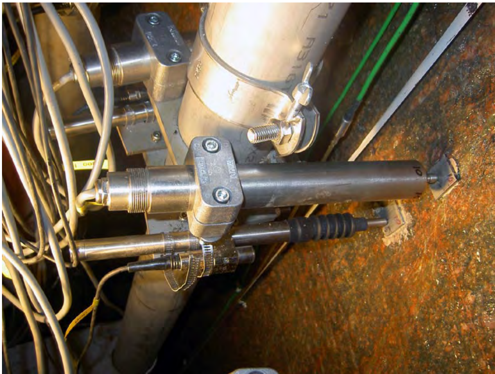
Figure 3-15. The new clamp. The top sensor is the short-range LVDT and the lower ones are the long-range LVDT sensors. Only the short-range sensors were fitted with the new clamp system.
