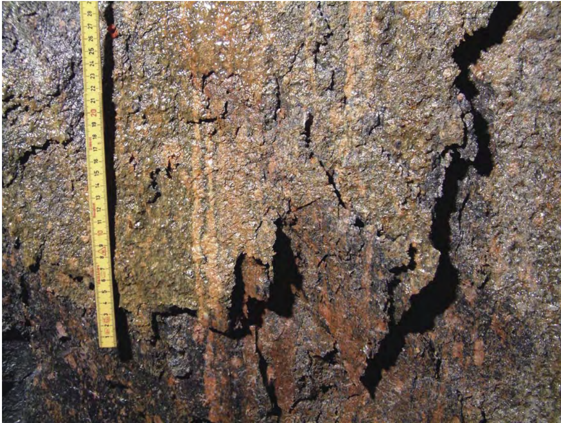
Figure 5-60. Photograph of rock wall at depth of approximately 4 m. The small cm-scale chips on top of the larger chips are clearly visible.
