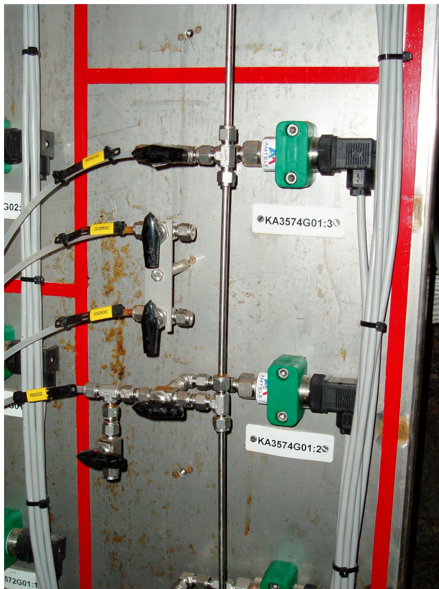
Figure 4-2 Pressure transducers connections
