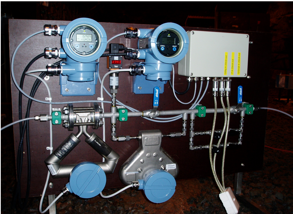
Figure 4-3 The equipment for flowrate measurement with Micro Motion Coriolis mass flowmeter system
