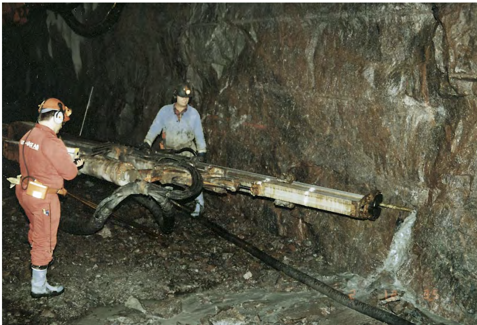
Figure 5-3. Penetration rate, colour of drill cuttings and water inflow rate were recorded during drilling.
