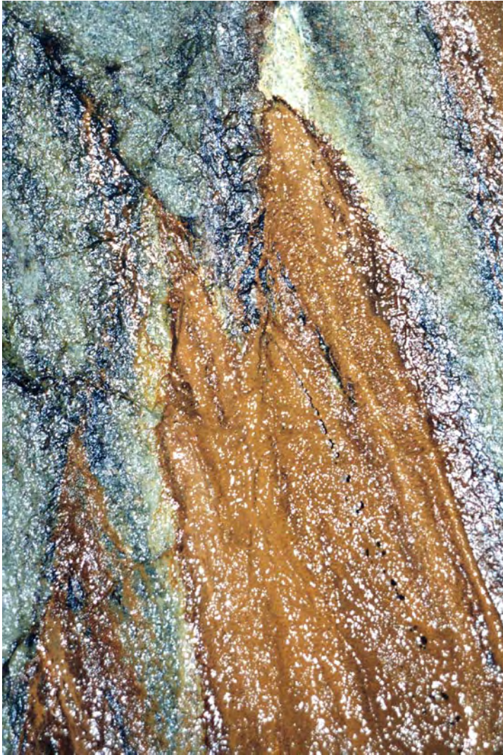
Figure 4-5. Photo from the TBM tunnel showing a point inflow of water. These kinds of distinct inflows are possible only in a TBM tunnel, where the flow paths close to the tunnel are not disturbed as in a blasted tunnel.
