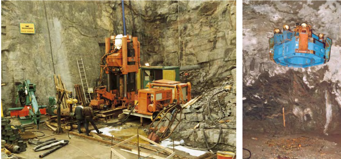
Figure 2-5. Raise boring of shaft. Drilling machine at the surface and the raise boring head at the -220 m level before drilling of the first shaft section.
