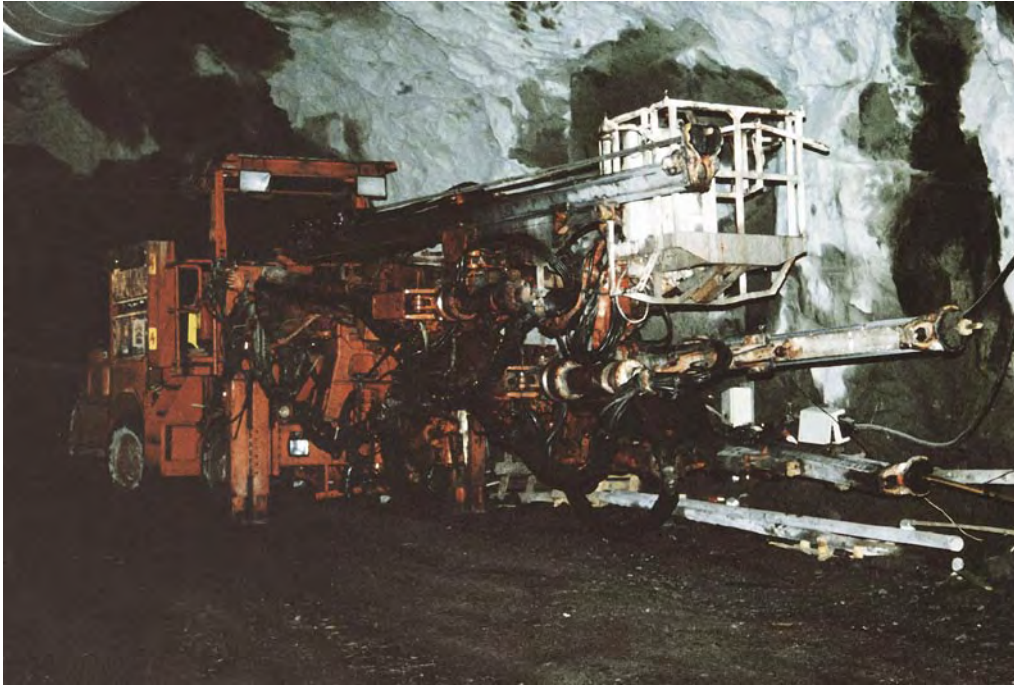
Figure 2-2. The drill rig used for drilling of blast holes and probe holes.
