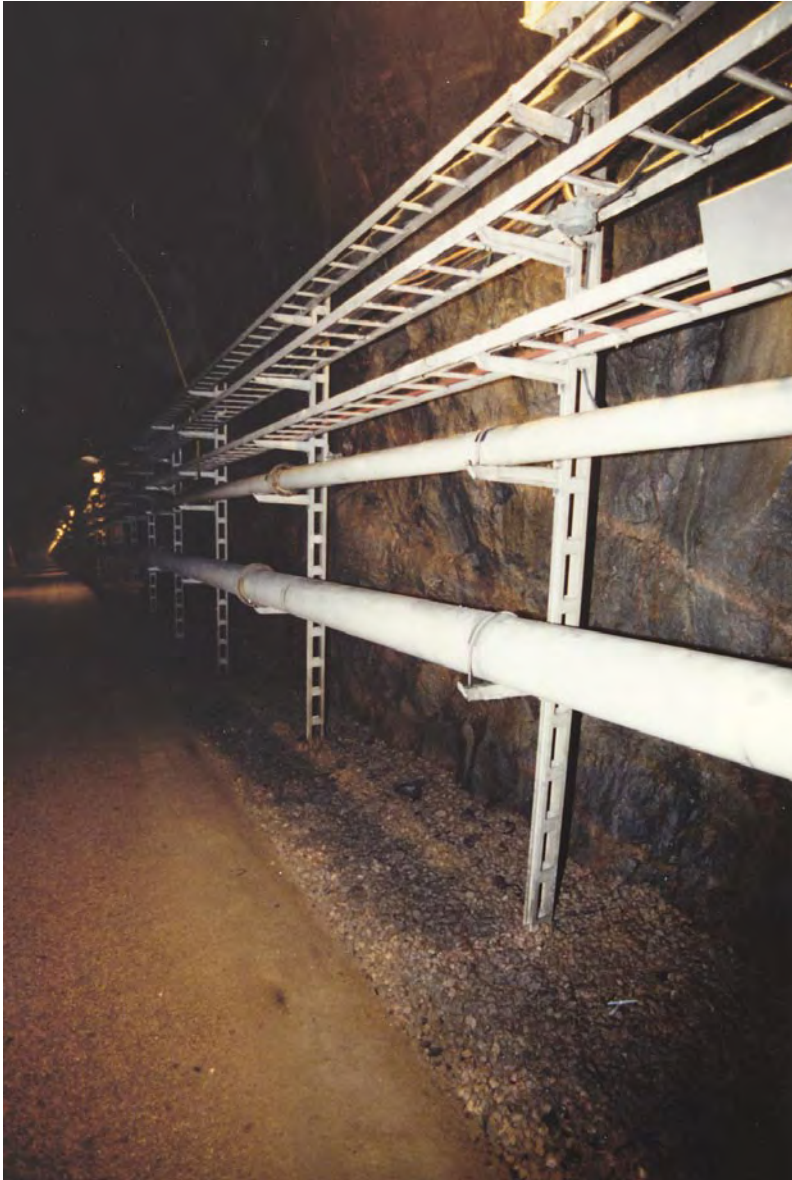
Figure 2-7. Pipes, cables etc installed on brackets on the tunnel walls.
