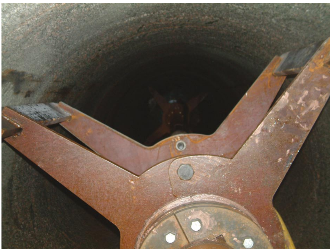
Figure 5-7. Wing-stabilizer used to centre the drill string and to avoid lateral buckling.
