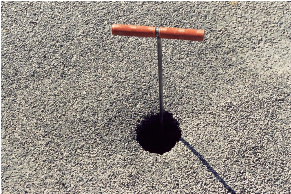
Figure 5-4. Damage to road surface caused by loss of underlying filling where the road crosses the lineament some 600 m west of St. Dalby. According to residents in the neighbourhood this problem has occurred on more than one occasion.
