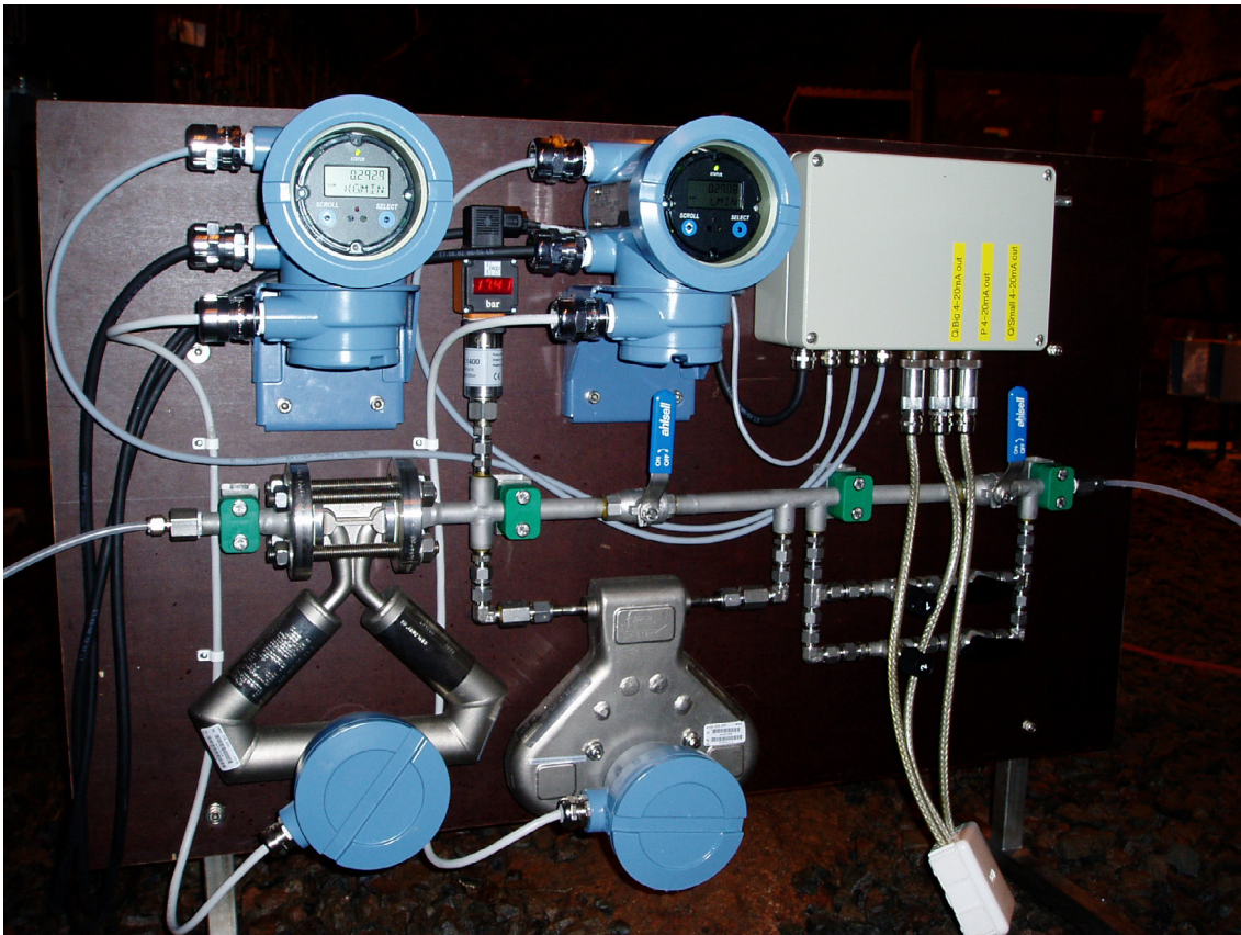
Figure 4-3 The equipment for flowrate measurement with Micro Motion Coriolis mass flowmeter system
