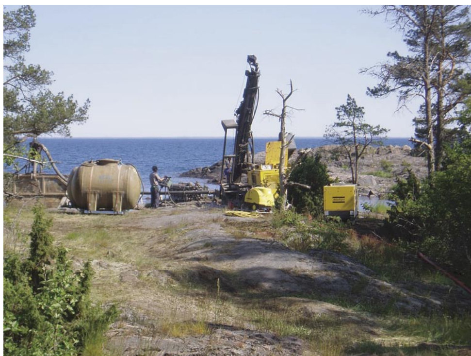
Figure 4-2. Drilling rig at the site for HAV11 on the south-eastern coastline of the island Ävrö.
