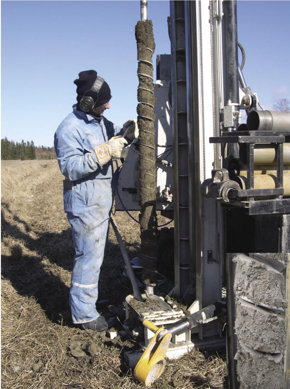
Figure 3-24. At the installation of groundwater monitoring wells, corings were performed using an auger drill. The coring sites are distributed within the investigation area and resulted in samples of higher quality than the percussion corer. The picture shows clayey till obtained from 4 m depth at Storskäret. Note the detail in the bottom right hand corner.
