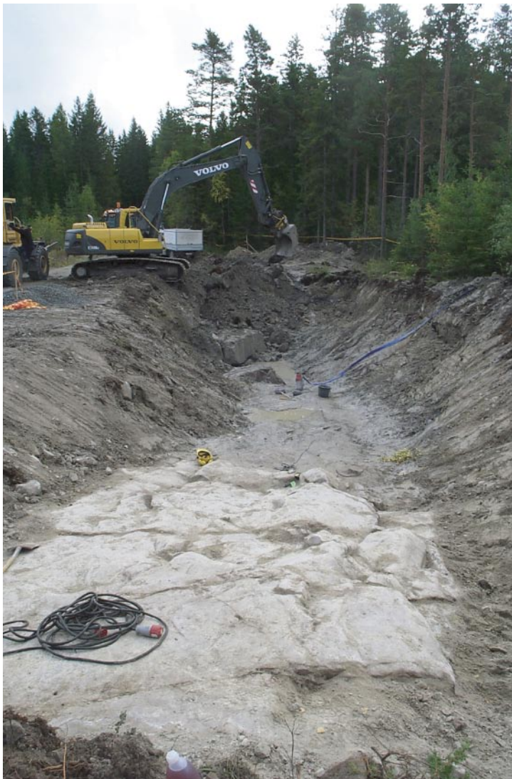
Figure 5-1. Photograph showing the trench LFM000811. The dark clayey till, Unit A, is located in the bottom of the trench.
