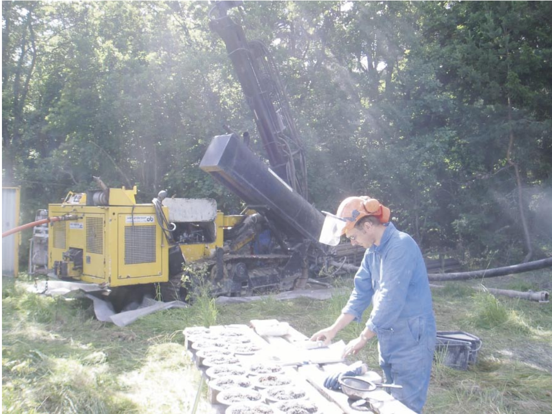
Figure 4-2. Drilling rig at the site for HLX17. The preliminary geological mapping can be seen in the foreground.
